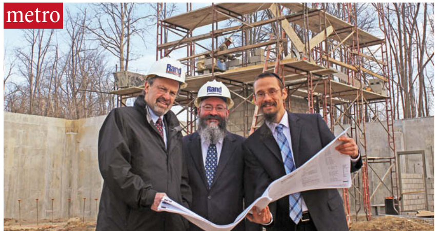
Fred Leeb, Rabbi Kasriel Shemtov and Dov Stein at the MJI construction site
